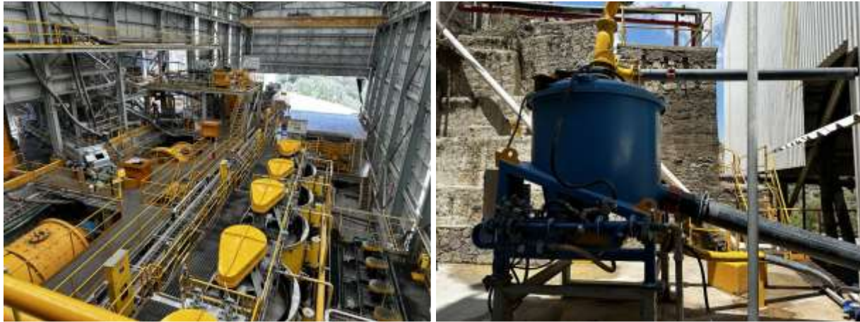
Figure 12.4 El Cubo Mines Complex Processing Plant (Left: view from control room; Right: Falcon centrifugal concentrator)
