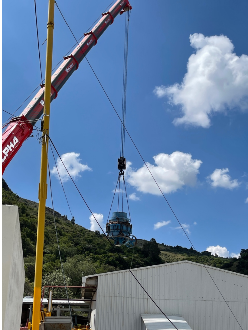
Crane winching one of two Symons 4.25ft crushers into the El Cubo mill
